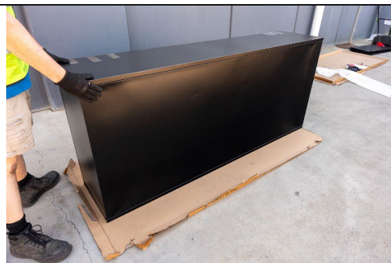
Fig. 31. Cabinet laid flat on its side.
